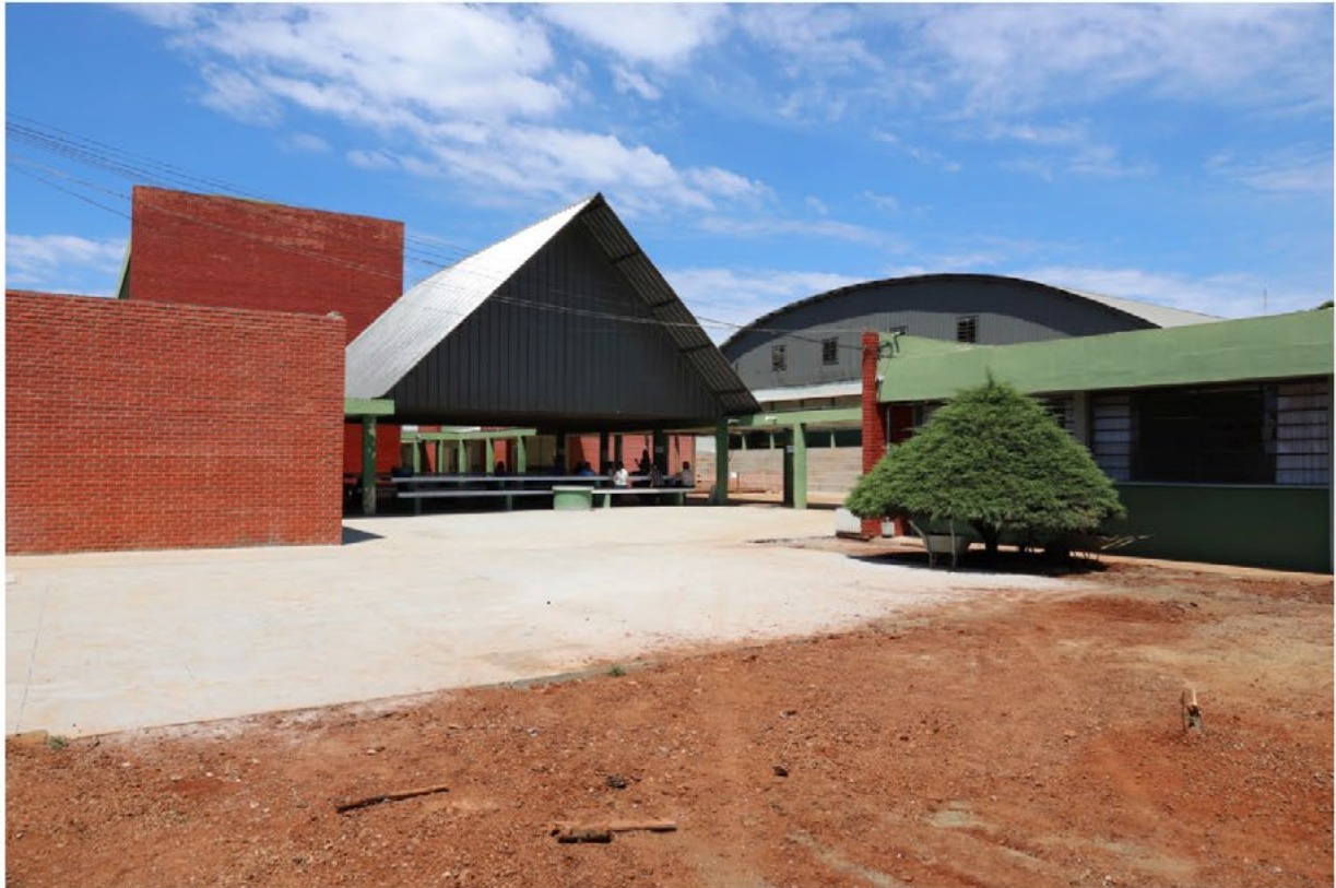
Work in the courtyard of the Wolff Klabin State High School in Telemaco Borba (Parana state). Photo: Klabin's archive
